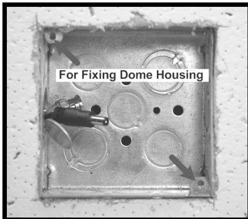
Figure: 4S Mount Electrical Box
